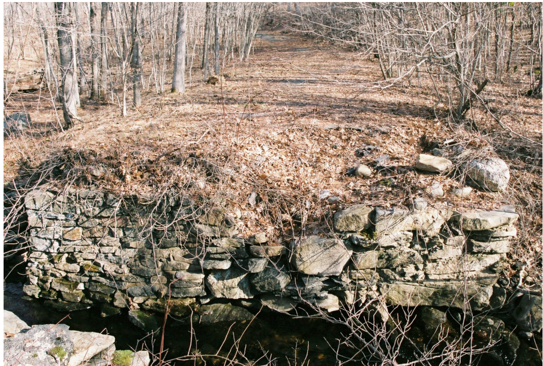
Figure 16. Bridge wall for road which is no longer in use near Site 4
